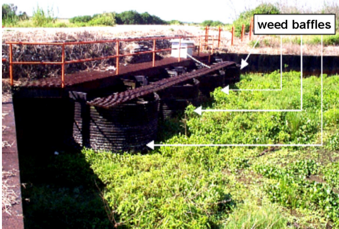
Figure 3. Debris baffle installed on canal culverts. Credits: P. Whalen
