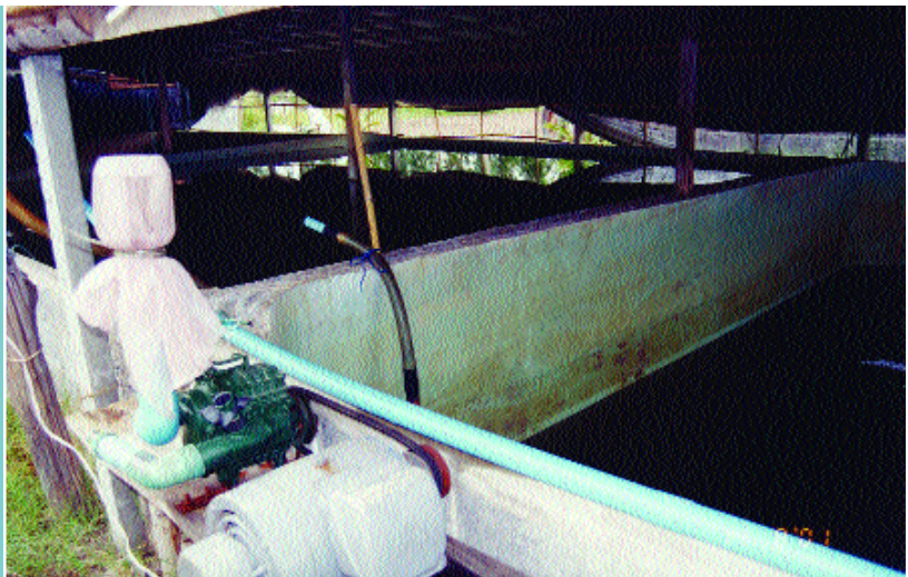
Figure 25 Tanks for storing hypersaline water and freshwater, and for mixing purposes at an inland hatchery in Thailand; note the roof and side covers for excluding aerial pollution and controlling temperature
