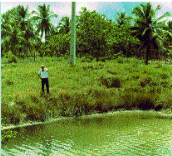
Figure 47 The bank of this freshwater prawn pond is being eroded because its slope is too steep (Hawaii)
