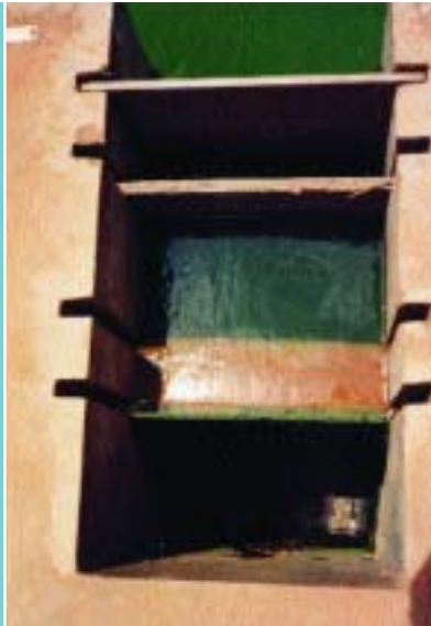
Figure 56 The outlet structure, sometimes known as a 'monk', can be used to control the level of the water as well as to screen the water to prevent the loss of freshwater prawns (Brazil)
