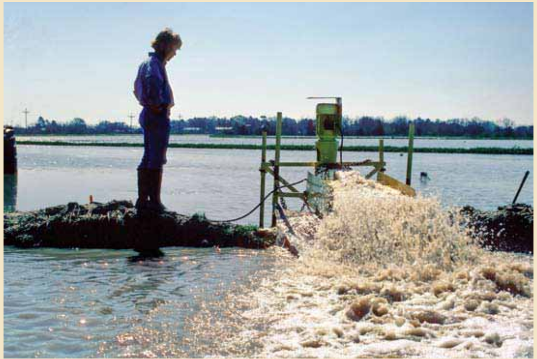
Figure 4.3. Many crawfish ponds can be adapted to allow for circulation using one or more re-lift pumps.
