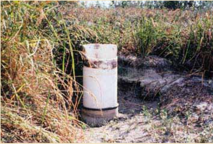
Figure 4.5. Drains must have sufficient capacity to lower ponds over a short period of time.
