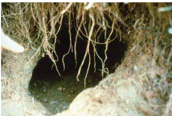
Figure 9.8. If left uncontrolled, burrowing rodents can cause costly damage to crawfish ponds, occasionally resulting in levee failures.
