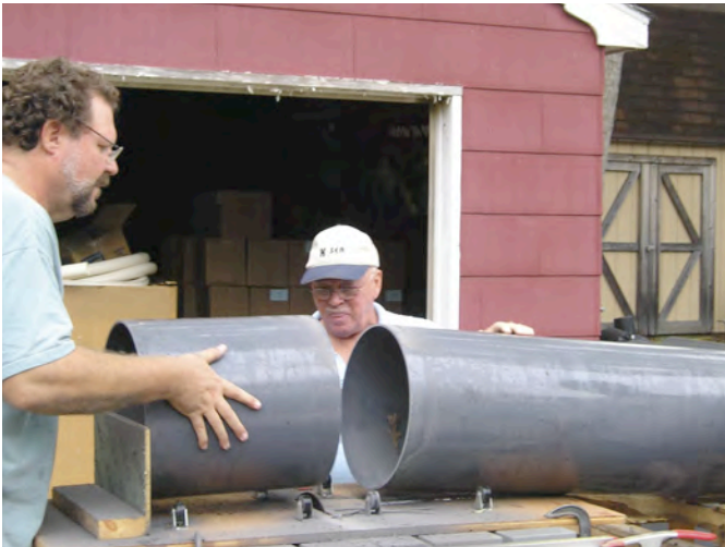
Figure 5. Sections are cut with the jig to make silos from the full length of pipe.
