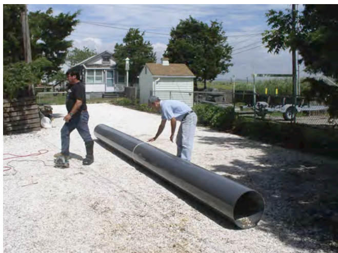
Figure 2. A standard length of 16" PVC duct pipe to be cut into silo sections.
