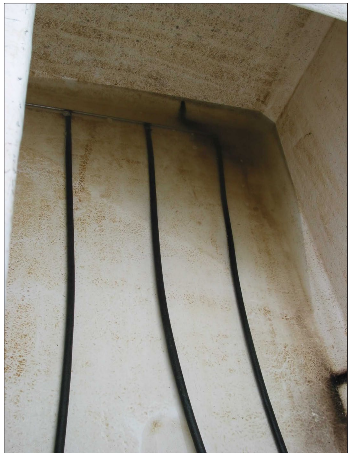
Figure 8. Diffuser hose grid on the floor of a fiberglass tank.
