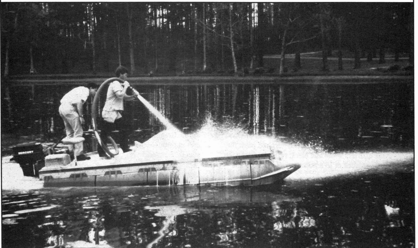
Lime application using a pontoon barge and water pump to evenly distribute the lime.
