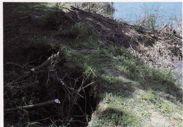
These beaver tunnels are in a man-made dam built to impound water. Such tunnels commonly cause failure of dams, loss of water and costly repairs.
