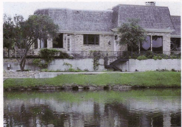
Beaver tunnels under walkways and houses, as shown here, can cause major structural damage if the tunnels collapse.
