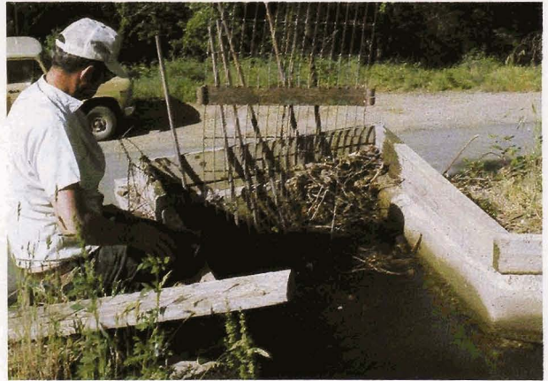
Beaver interfered with crop irrigation by plugging this headgate with sticks and mud.
