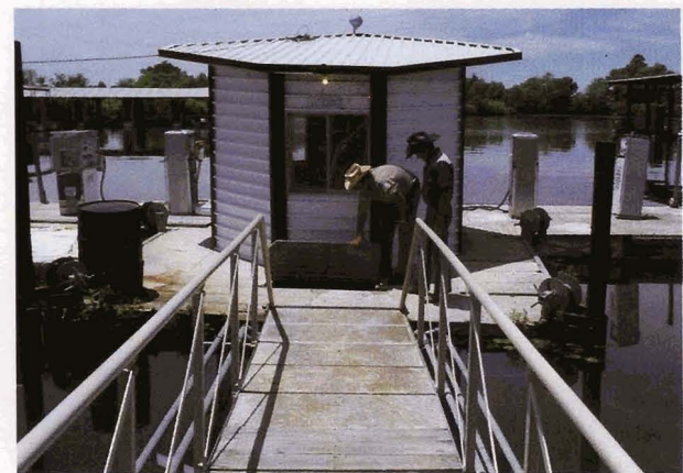
Damage to the flotation supports cause the houses and docks to tilt or sink; repairs are quite expensive.
