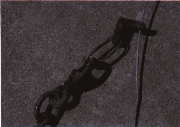
The angled slide wire lock holds the chain at the bottom of the pond.
